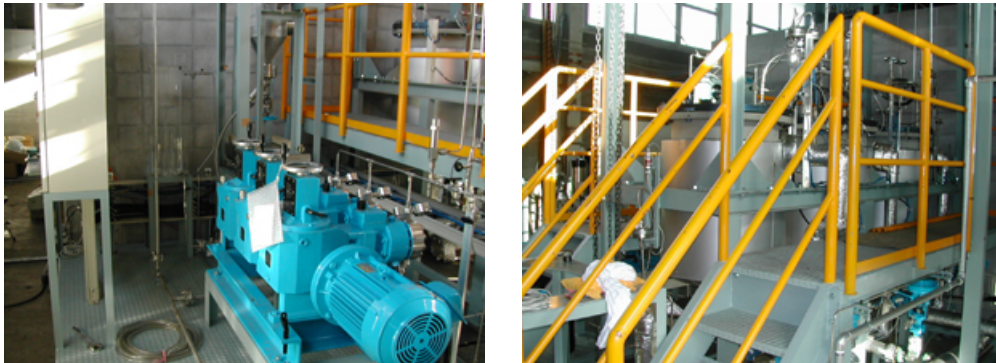
Figure 3. Photographs of CWS vaporizer system
